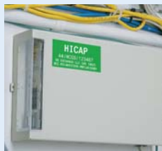
Control Panel Labelling
