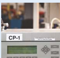
Control Panel and Electrical Panel Labels
