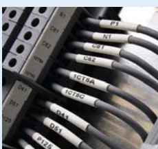
Wire & Cable Marking
