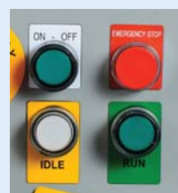
Control Panel Labelling
